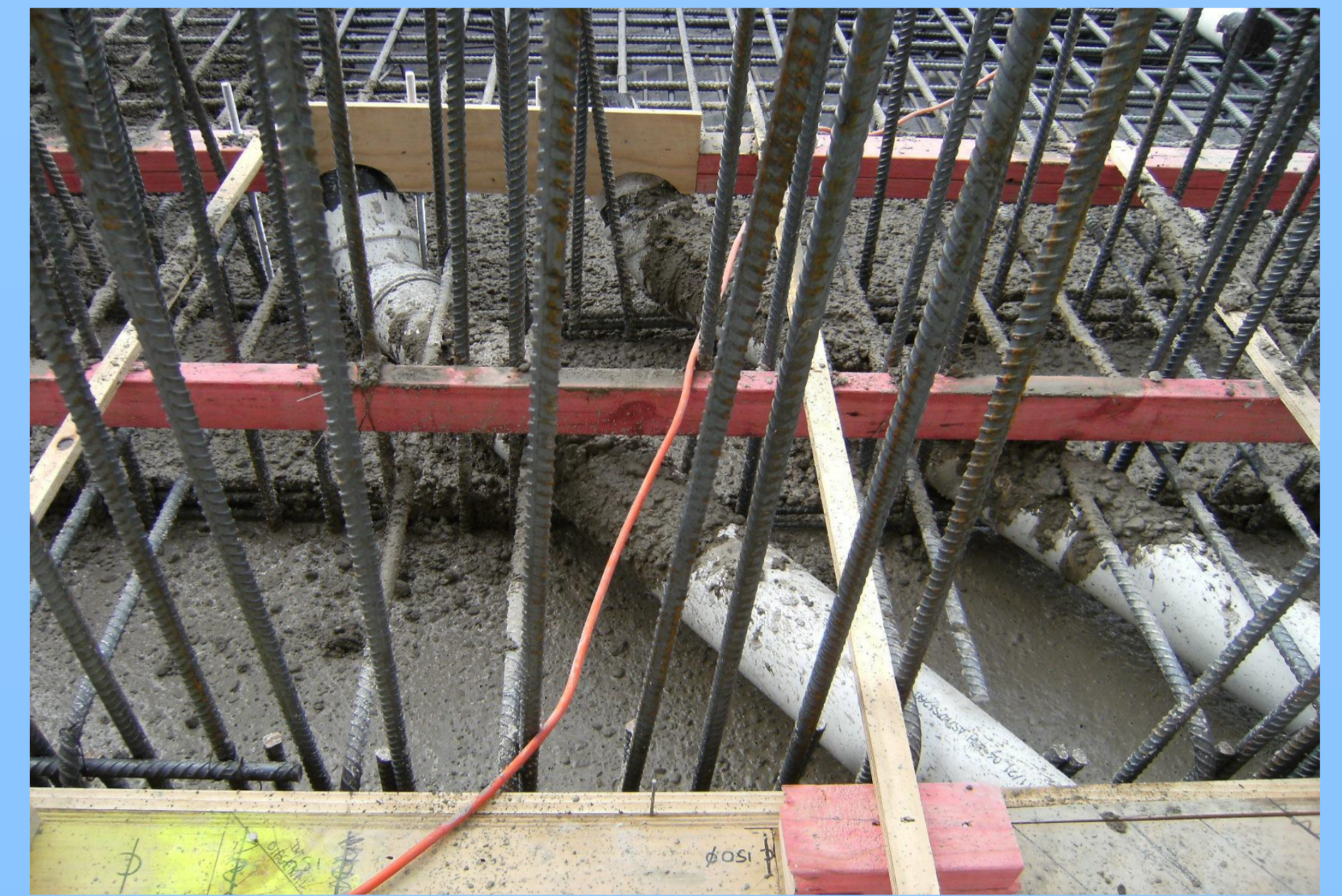
Photo 3 - Penetrations such as ducts for service supply present in secondary barriers
