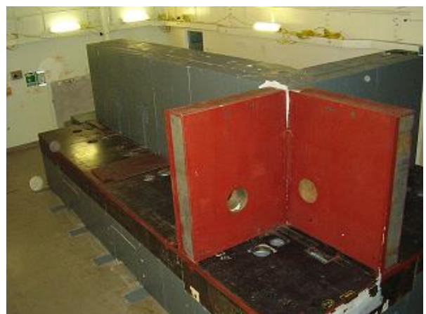
Figure 4(b) Cells nearly demolished
