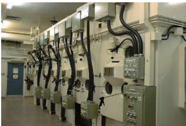
Figure 4(a) Cells in place
