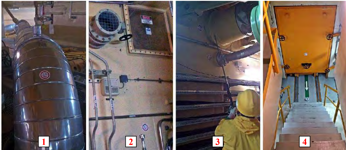
Figure 2: Some selected RBP's: 1=live steam line above Steam Generator in level +18.80 m; 2= rupture valve at level +5.00 m; 3= penetrations belonging to level +0.50 m; 4= door giving access to components of the moderator system in level -12.00 m
